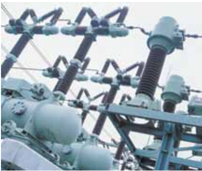
Safe energy production with Schunk plug-in brush holders. Photo: KKW Marl
